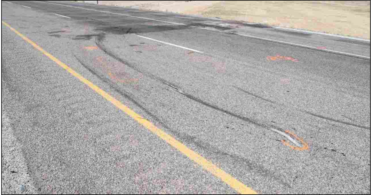
Figure 2.2 Example of a roadway gouge caused by a wheel rim
