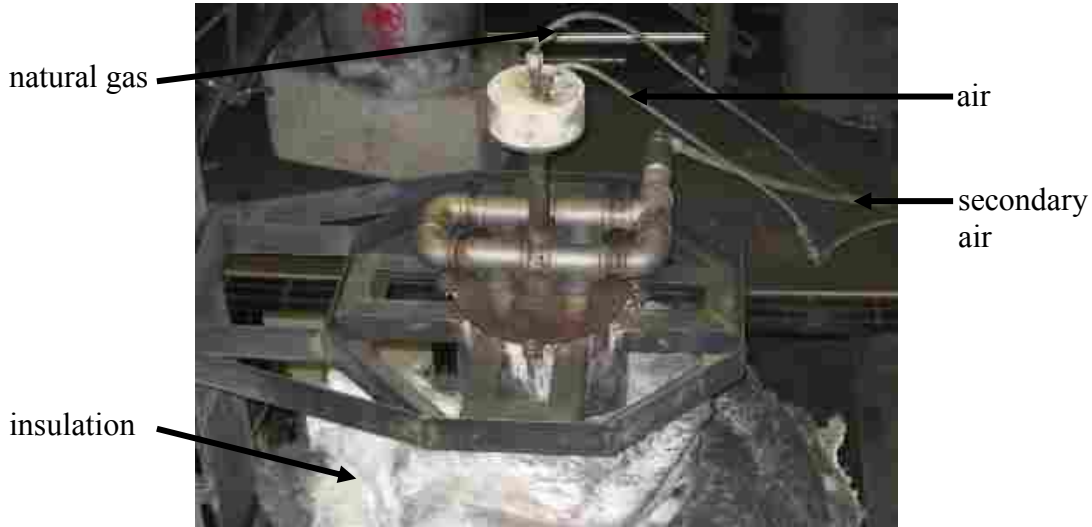
Figure 3-3. View of the top of the reactor, which includes the preheat burner system.
