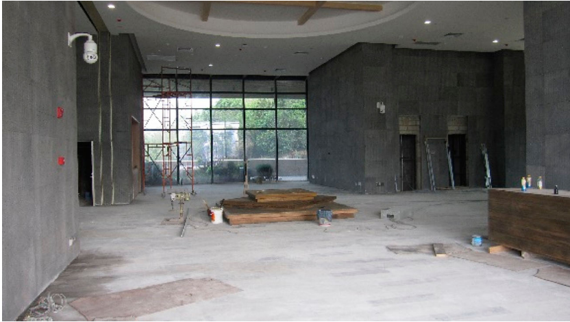
Image 3. The unfinished lobby of a museum that was to open to the public in two weeks. The rapid pace of local government contracts shaped Jiangnan Design's pace of growth. Photo by author.
