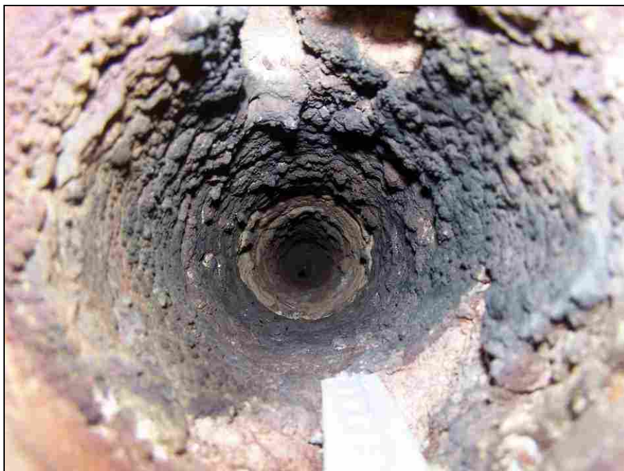
Figure 32. Looking down into the MFR with the burner removed reveals ash deposits with colors characteristic of the oxidizing and reducing conditions in different regions of the MFR.
