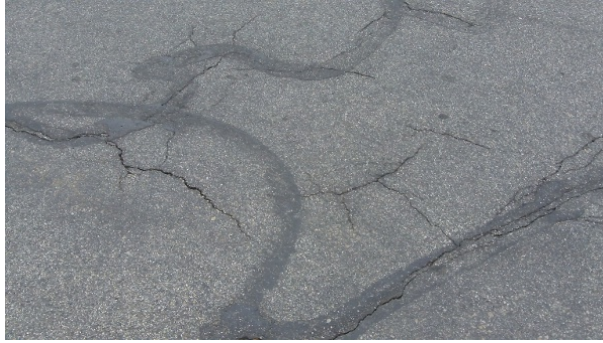
Figure 4-4: Photograph from Street Cracks Problem-Finding Item
