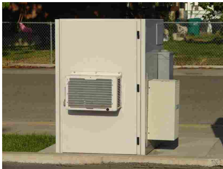
Figure 10 – iProvo Demonstration Area Cabinet
