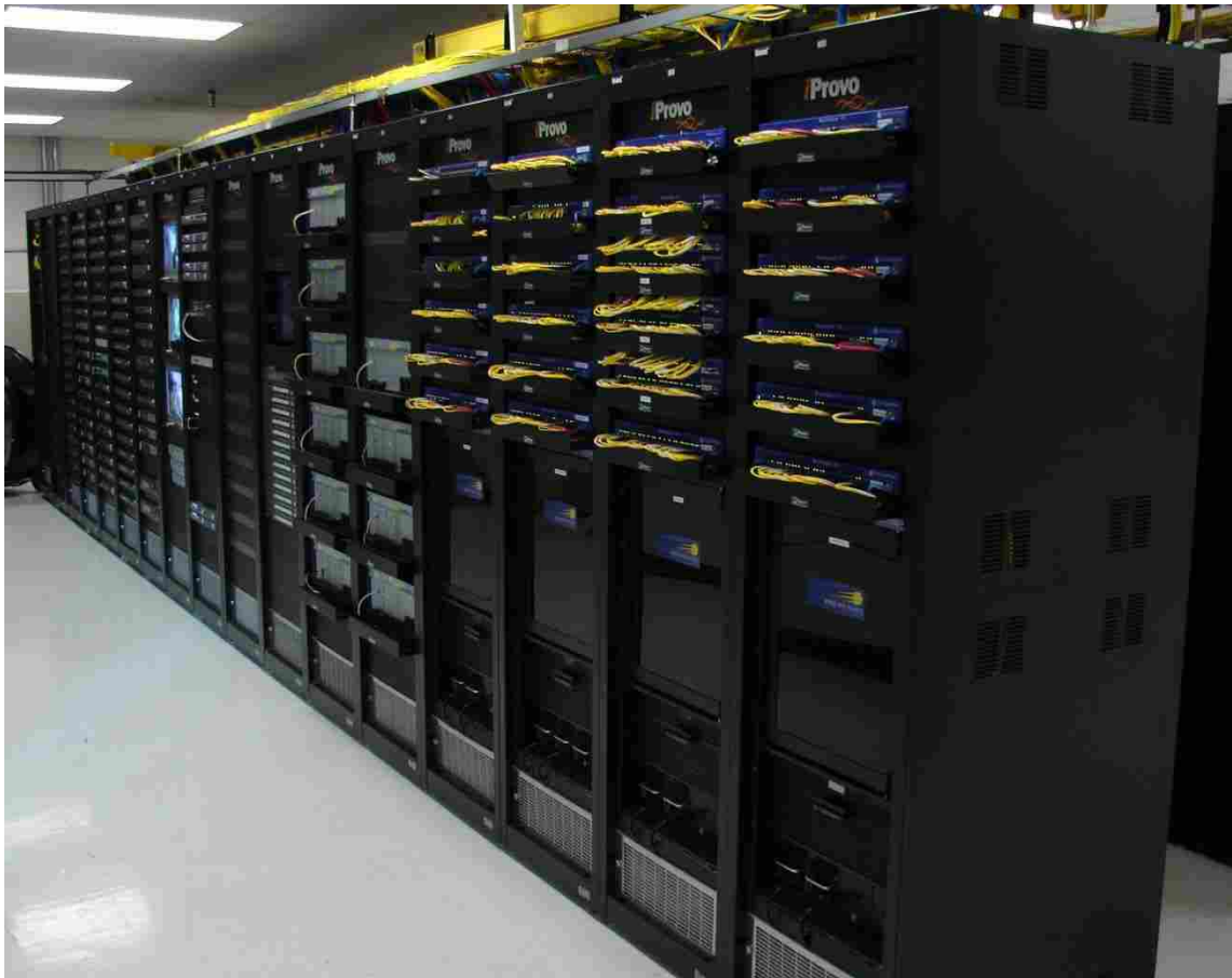
Figure 28 - Provo Network Core and Headend
