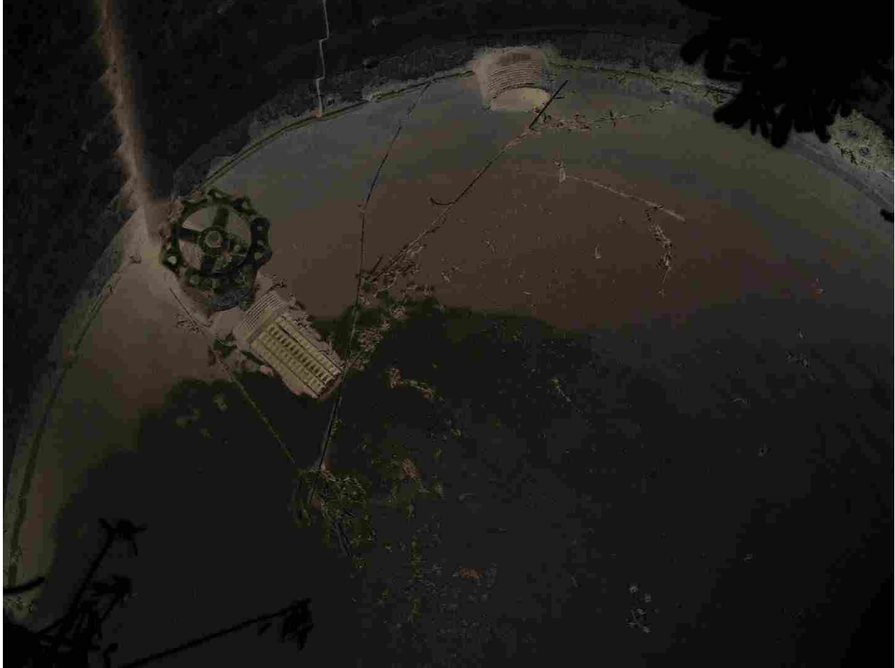
Figure 1.9. Interior of a springbox showing the pair of pipes that funnel water away from the spring source. One pipe, the outflow, diverts water to a cattle trough installed away (50-800 m) from the wet meadow. The other pipe discharges excess water out in the original wet meadow.
