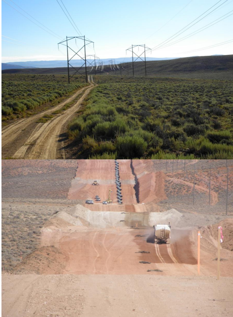
Figure 2-2. Images depicting pipeline right of way (ROW) at the study site where we evaluated pygmy rabbit ( Brachylagus idahoensis ) response to construction of the Ruby pipeline in northern Utah, USA 2010 – 2012. Images of ROW before (top) and during (bottom) construction.
