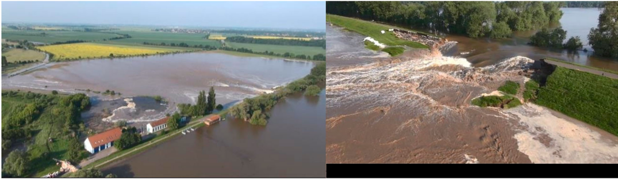
Figure 5. Left: overview photo of the inland while the flooding evolves, Right: overview photo of the breach at 10-jun-2013 (Grubert 2013; Weichel 2013).
