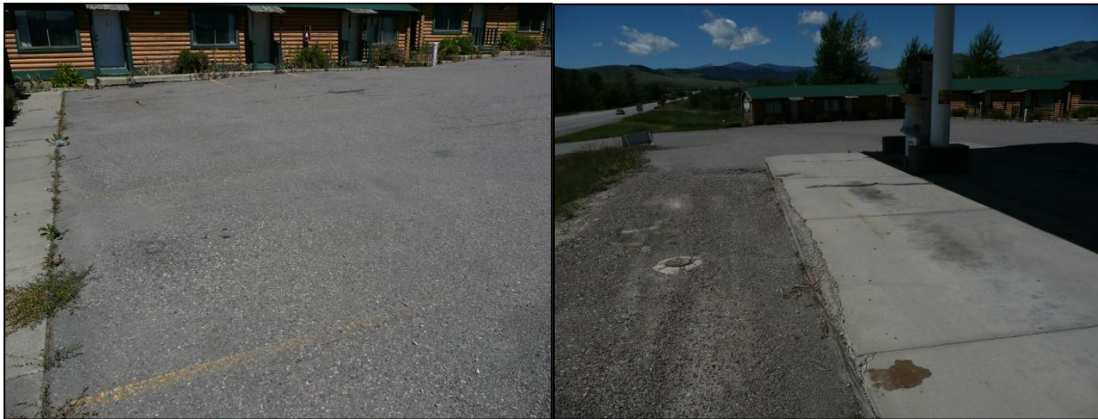
Figure 4. Views of the Paved Asphalt Parking Lot and Concrete Pad with Staining
