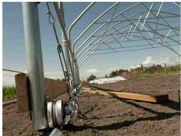
Part of preparation for next season is the construction of this moveable hoop house at 13 Mile. The hoophouse will protect vegetables from inclement weather.
