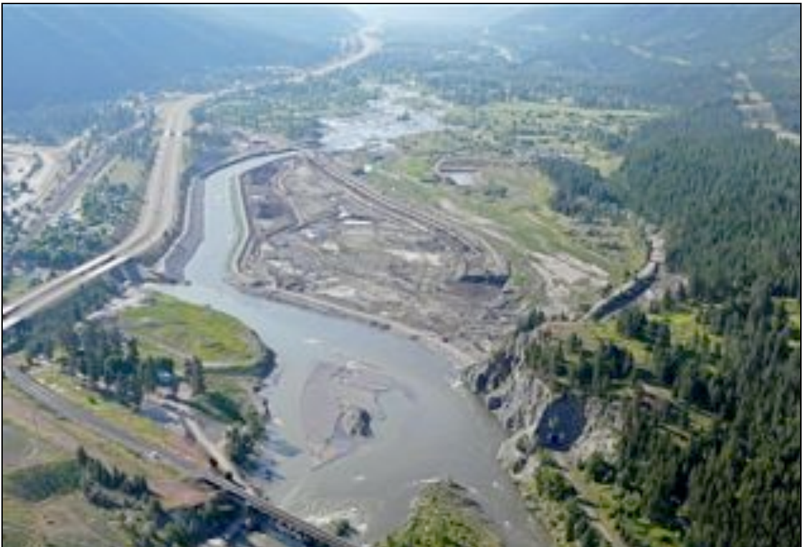
The same view in June 2009, after the removal of the dam and contaminated sediments behind it. Courtesy of CFRAC.
