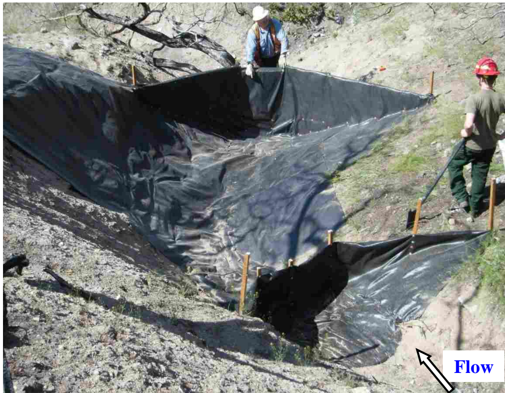
Figure 8. Tandem sediment retention structures in the channel. Geotextile woven fabric was secured to the up-channel face of the framed structures and extends up-channel attached with sod staples to the bed and banks. Tandem structures increased the maximum sediment storage capacity of sediment retention structures. Photo looks down-channel.
