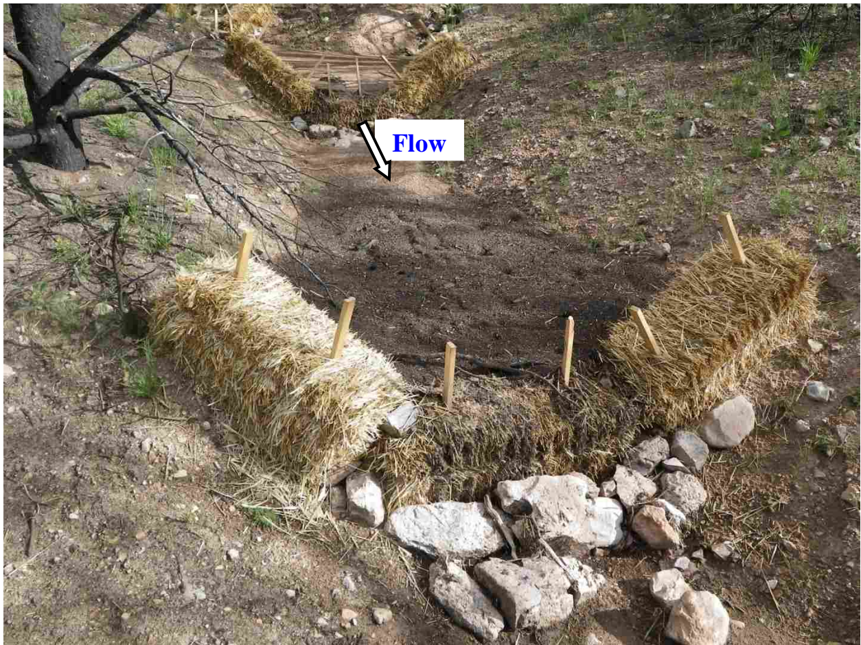
Figure 17. Straw bale check dam in catchment G filled to capacity during a 11 mm (0.4 in), 13 mm hr -1 (0.5 in hr -1 ) I 30 intensity rain event on 8 Jul 2011, which is less than a 1-year return period I 30 intensity event. Spillway rocks to reduce scour were undisturbed by flow. Photo looks up-channel.
