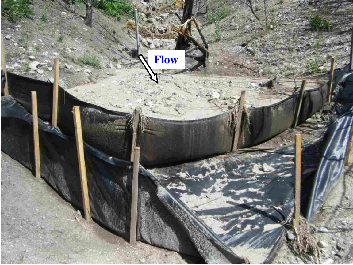
Figure 12. Sediment overwhelmed the upper sediment retention structure and caused the lower sediment retention structure to fail in catchment F from a high sediment yielding 16 mm (0.6 in) 1-year I_{30} 21 mm hr -1 (0.8 in hr -1 ) return period event on 8 Jul 2011. Overwhelmed and failed fences occurred only in Sevier Canyon due to the high sediment erosion rates during 2011. The reliable sediment yield is the measurement of sediment in the upper fence shown here, and is a conservative estimate of the true sediment yield from the catchment during the rain event.
