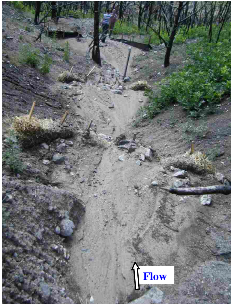
Figure 16. Channel F treated with 2 straw bale check dams that filled to capacity and were overwhelmed by a 16 mm (0.6 in), 21 mm hr -1 (0.8 in hr -1 ) I_{30} intensity 1-year return period event. The majority of sediment trapped by straw bale check dams was a sandy loam, but large woody debris and cobble mobilized by overland flow were also trapped. Photo looks down channel.
