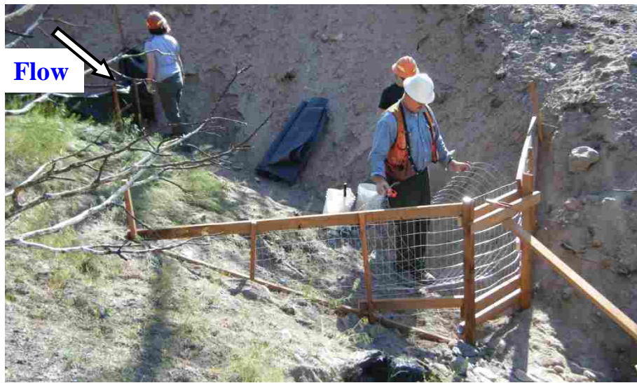
Figure 7. Lumber framing of sediment retention structure secured into the channel bed and banks with the added strength of wire mesh attached to the up-channel face. Spillway wall is located in the center of the structure with side walls opening up-channel. Photo looks up-channel.
