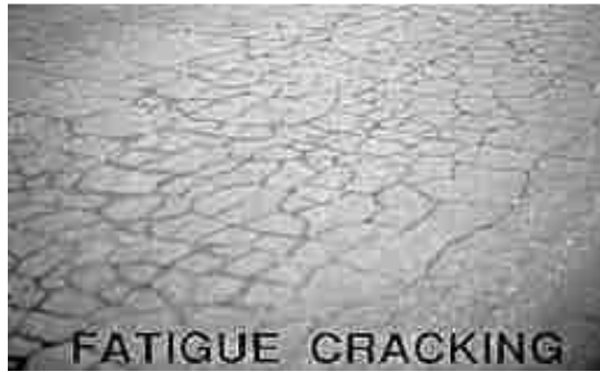
Figure 4. Fatigue cracking in an asphalt road surface [11].
