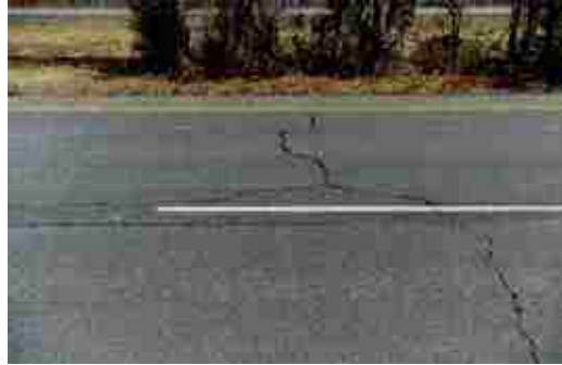
Figure 5. Longitudinal and transverse cracks due to thermal effects [11].
