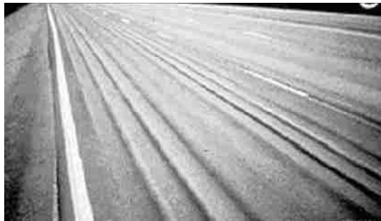
Figure 3. Severe ruts in an asphalt pavement [11].
