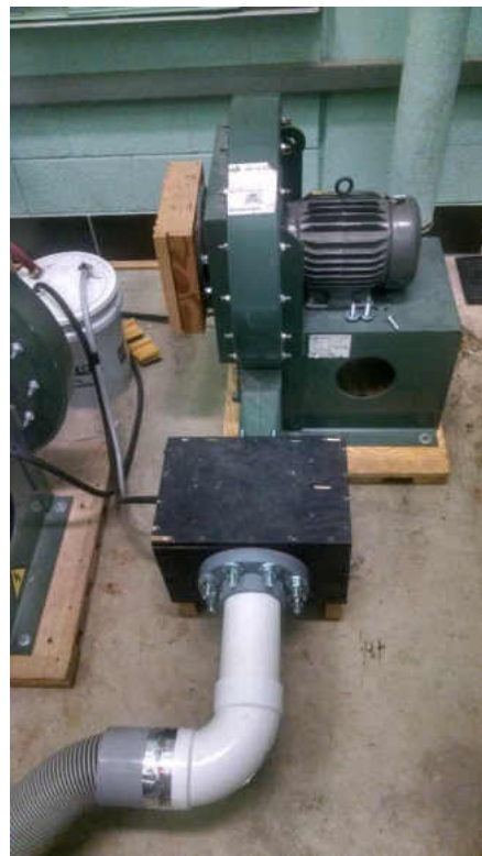
Figure 61. Endwall blower and heat exchanger
