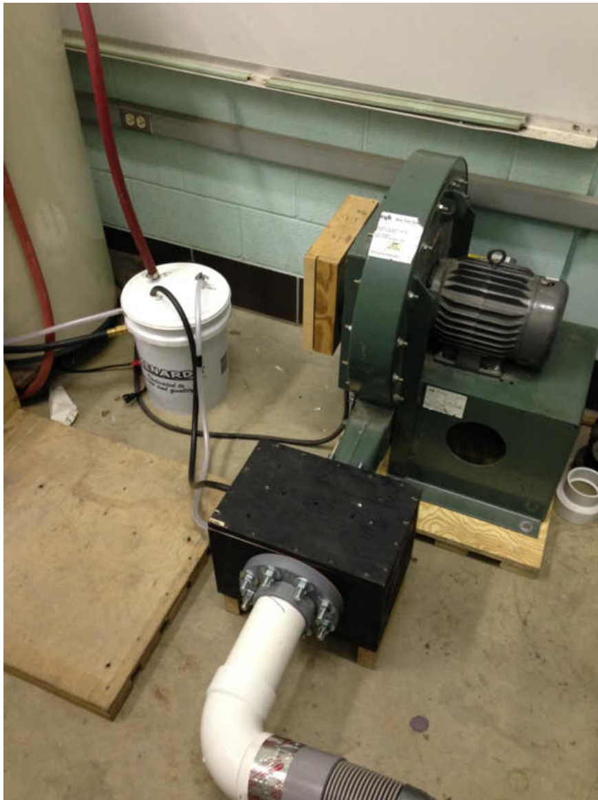
Figure 23. Small blower with new heat exchanger system.
