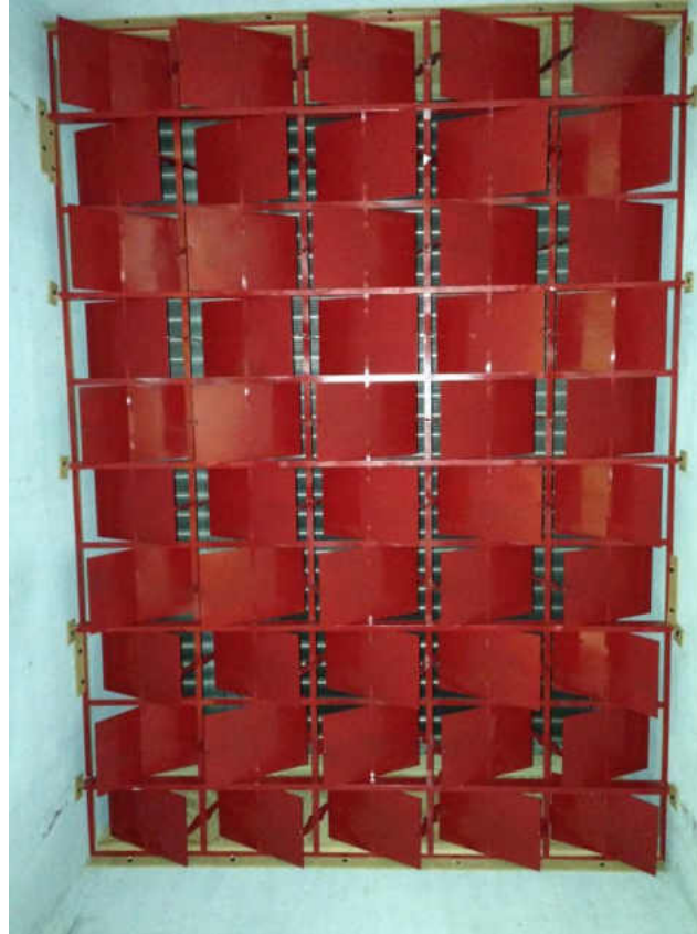
Figure 4. Flow mixer installed downstream of heat exchanger.
