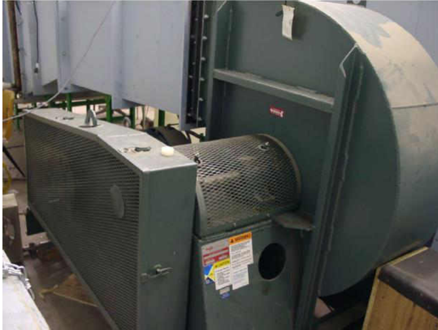
Figure 2. New York Blower used for wind tunnel [42].
