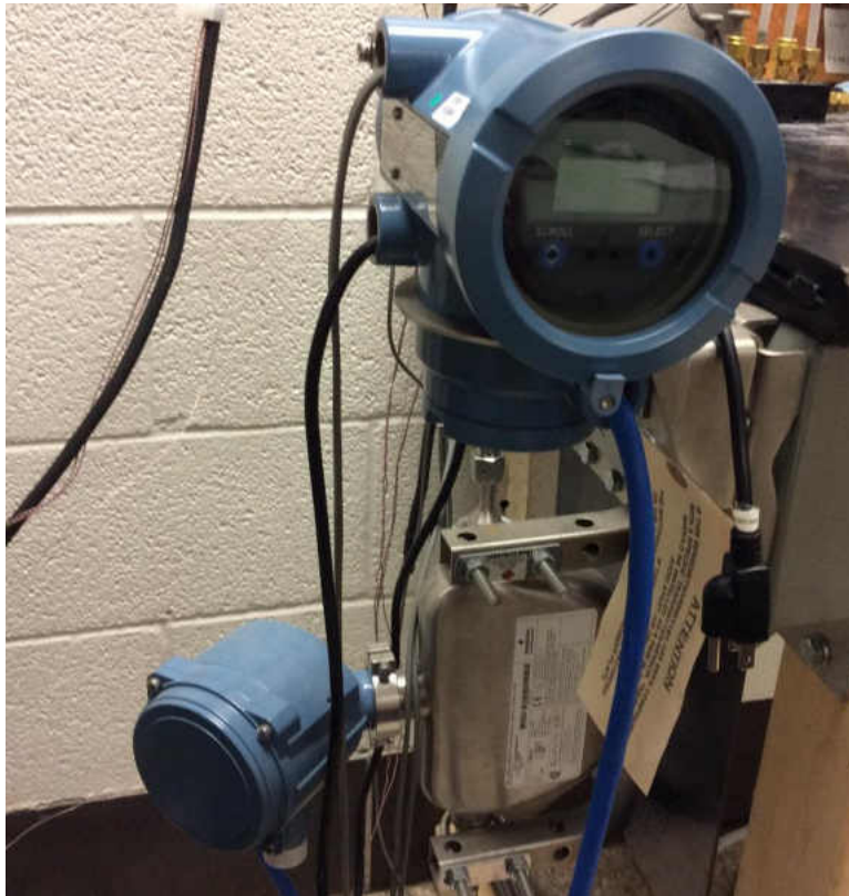
Figure 33: Mass flow meter
