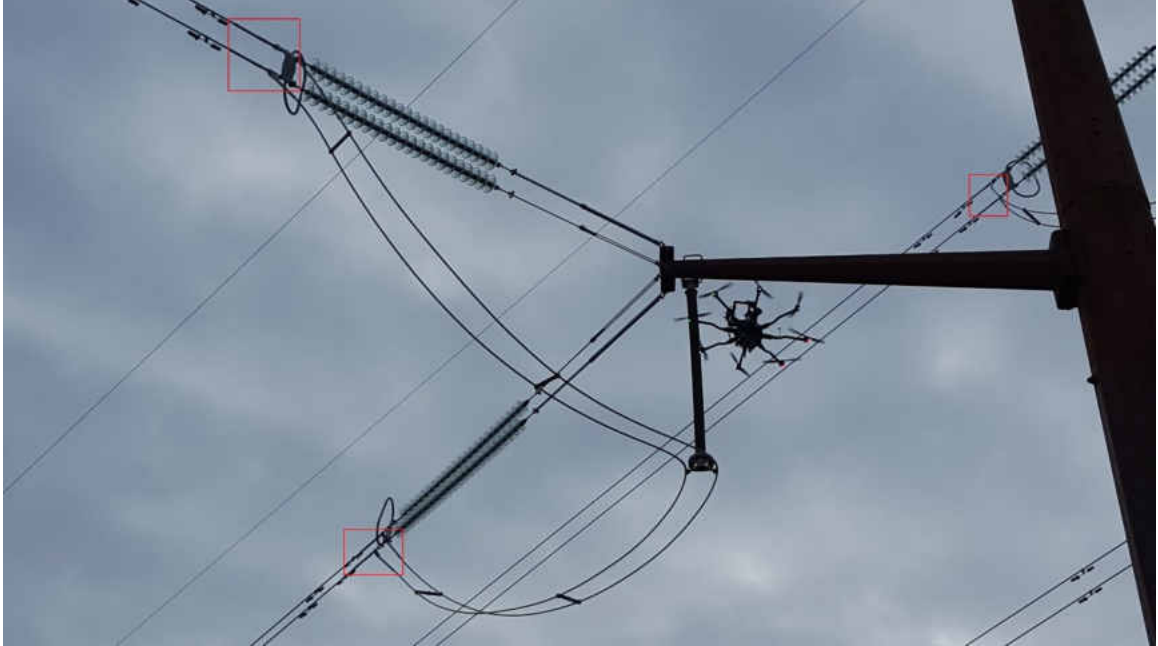
Figure 2: Image of UAS collecting DEBC inspection images. Regions in red contain DEBCs.
