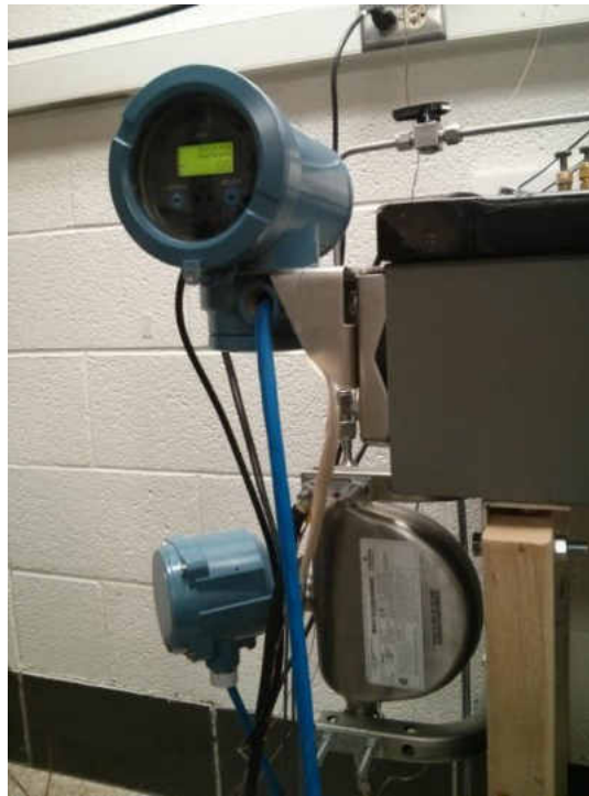
Figure 3.8: Micro Motion mass flow sensor connected to a 1700R transmitter.
