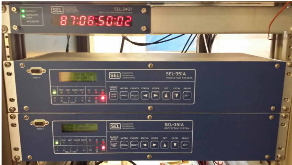
Figure 55. Front View of the PMU Equipment.
