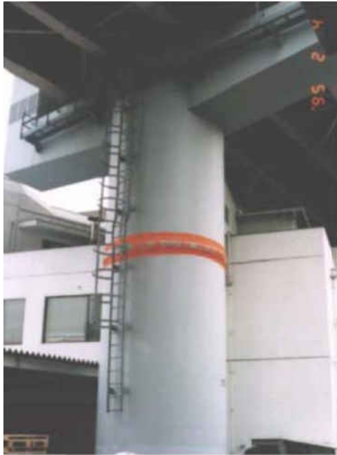
(a) Local Buckling
