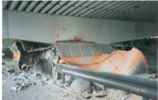
(b) Full Collapse.
