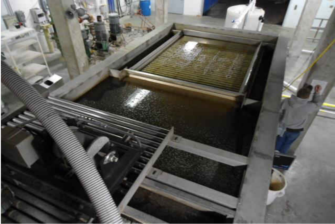
Figure 4.5.1.3. Top view of the MRI pretreatment unit.
