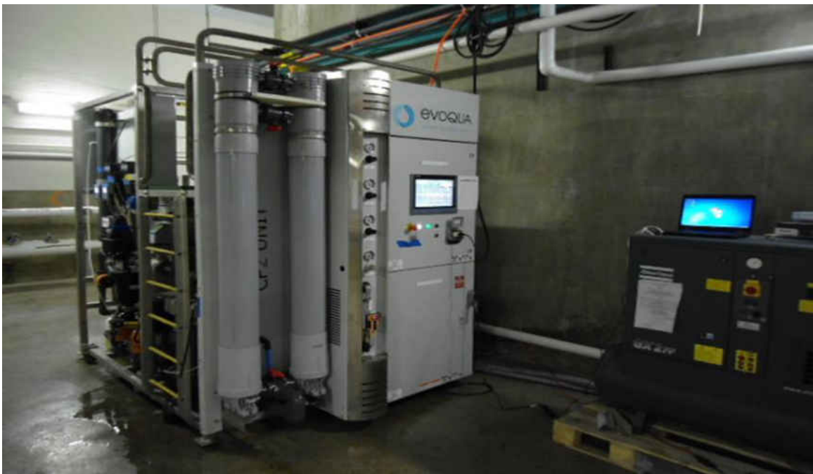
Figure 4.5.3.1. Front view of the ultrafiltration unit from Evoqua.
