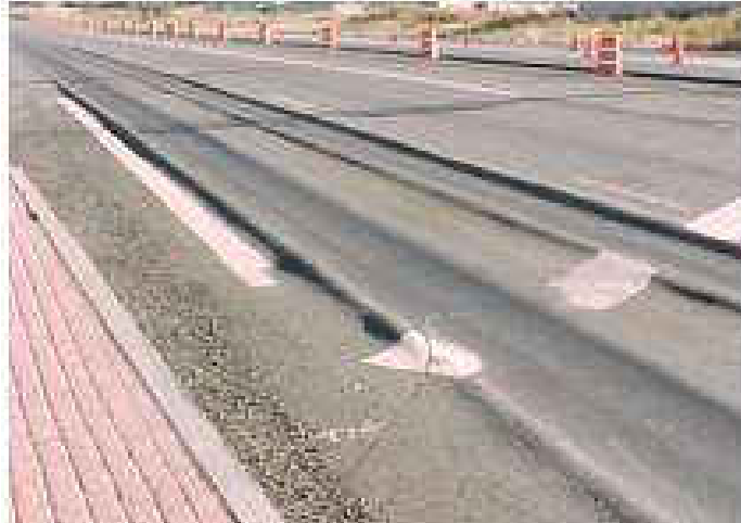
Figure 1. Rutting in a two-lane Asphalt Pavement (Pavement Interactive, 2009)
