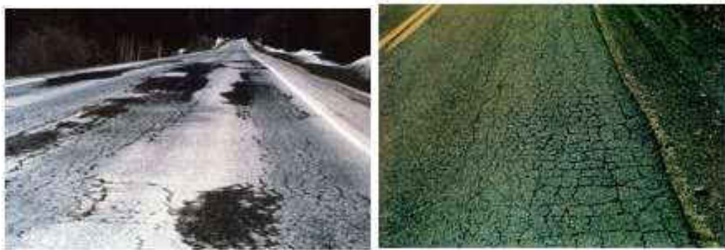
Figure 4. Images of Fatigue Cracking in Asphalt Pavement (Pavement Interactive, 2009)
