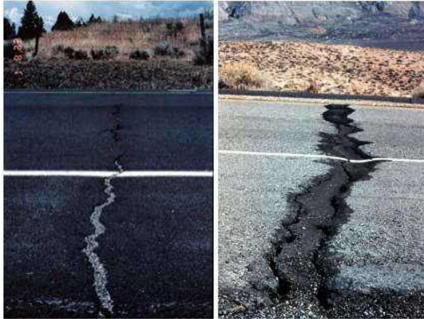
Figure 5. Images of Thermal Cracking in Asphalt Pavement (Pavement Interactive, 2009)
