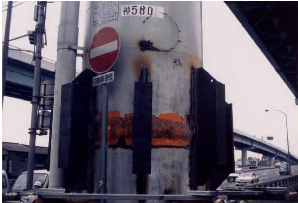
Figure 2. Damaged Bridge Pier Due to January 1995 Kobe Earthquake, Japan.
