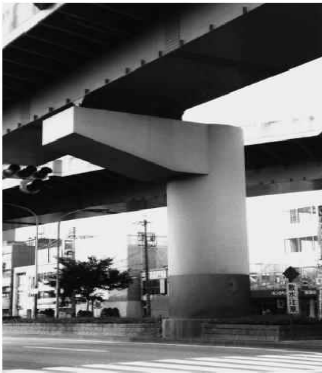
Figure 10. View of Eccentrically Loaded Steel Circular Section Bridge pier Constructed in Urban Area of Japan.
