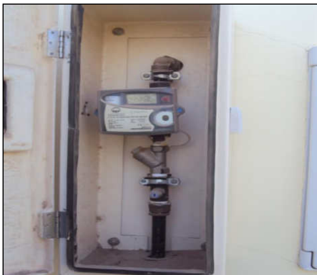
Figure 3.2: Water meter connected in houses in the study area (source: AADC)
