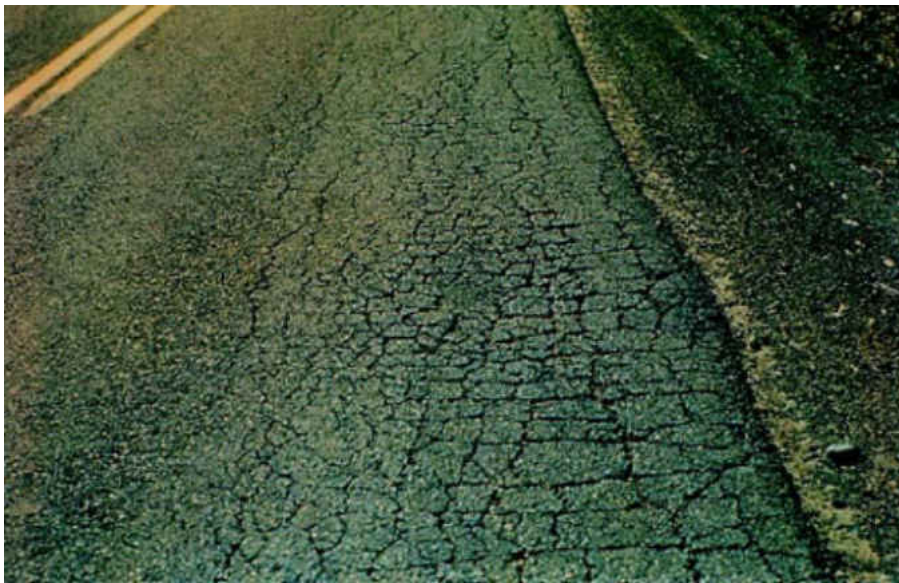
Figure 2.3. Very severely fatigued cracked pavement(PavementInteractive, 2019a)
