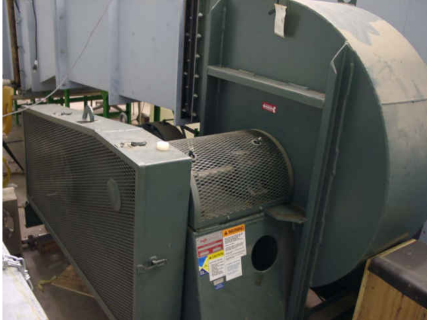
Figure 10. Blower used by UND.
