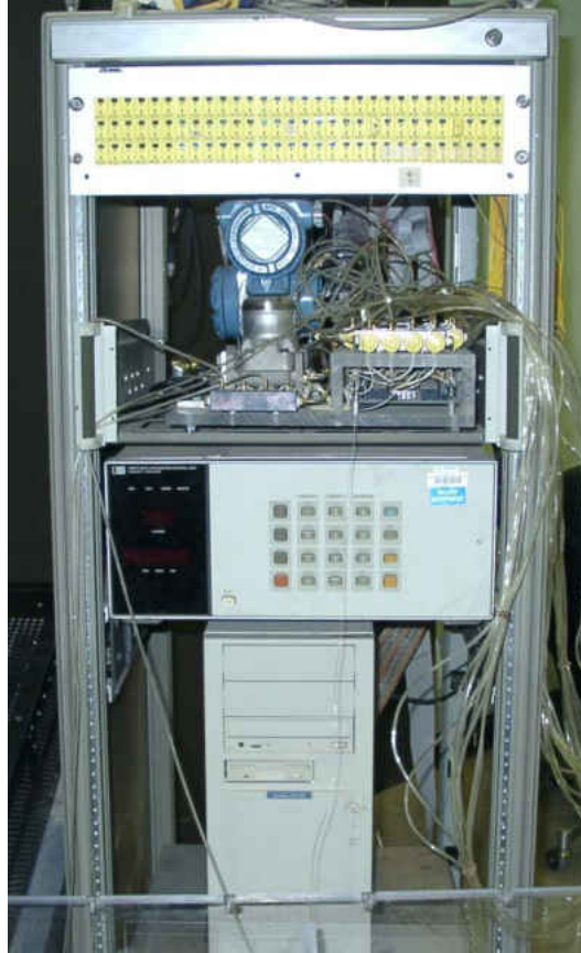
Figure 40. Stand containing the computer, HP unit, transducers, solenoids, and thermocouple jack panel.
