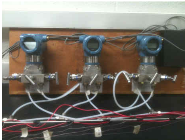
Figure 3.8. Three Rosemount pressure transmitters (model 3051) connected in parallel.
