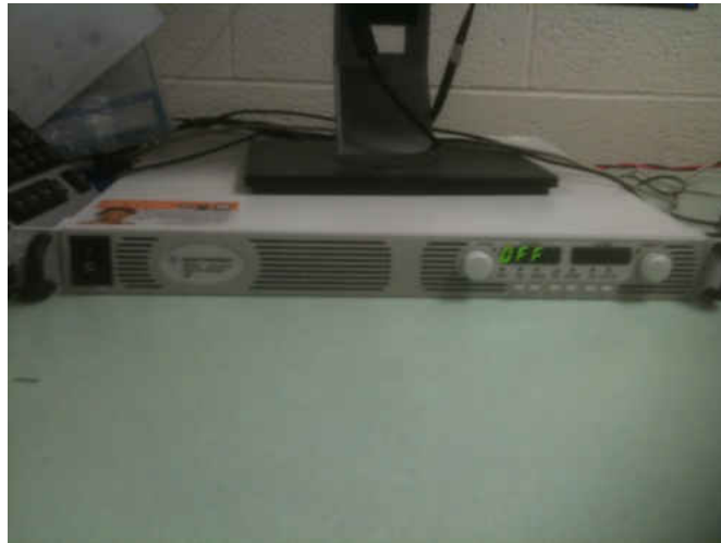
Figure 3.11. N5761A Agilent DC power supply unit.
