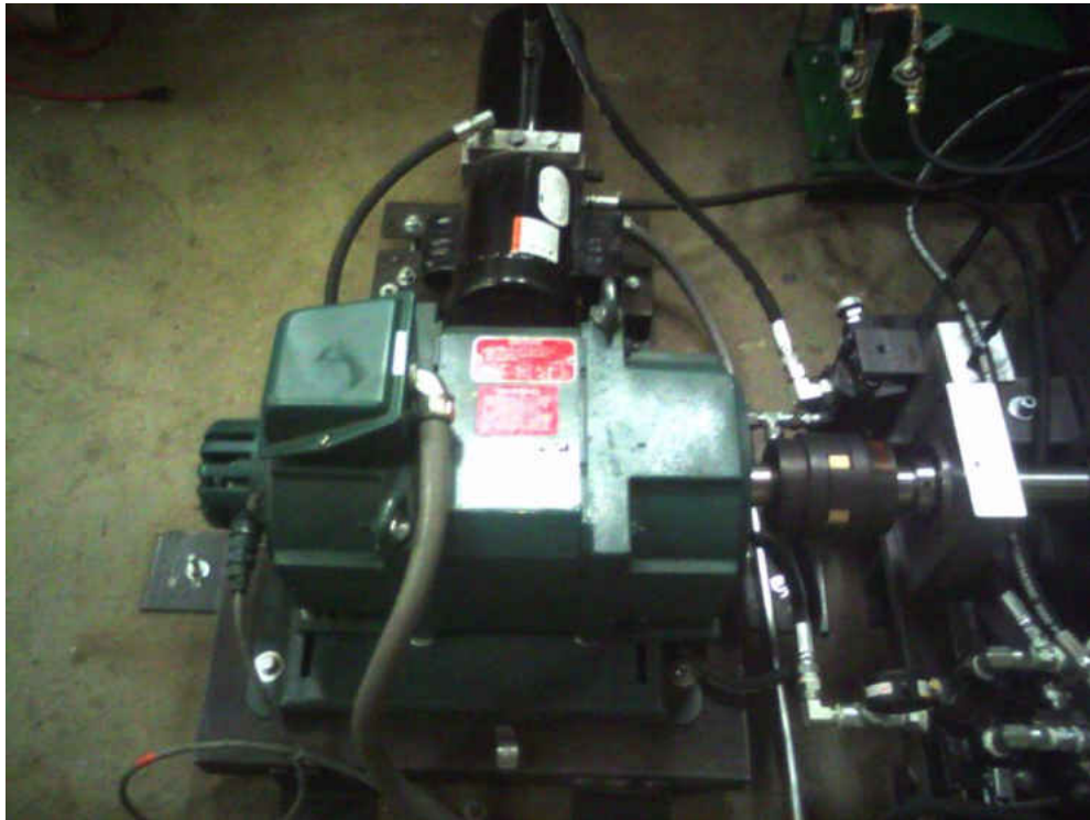
Figure 11 Allen-Bradley 10 hp Motor
