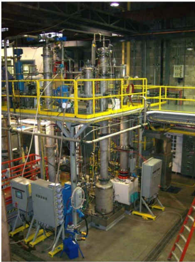
Figure 15. SASC system as tested during shakedown.
