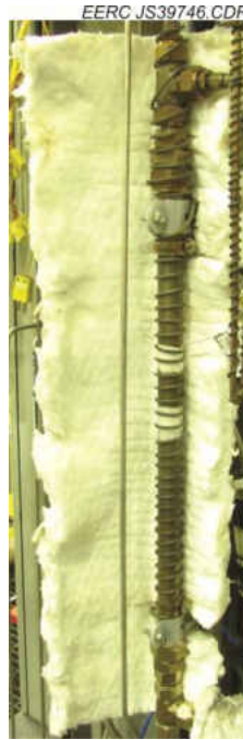
Figure 3.3. SS1 Membrane Mounts and Heat Trace.
