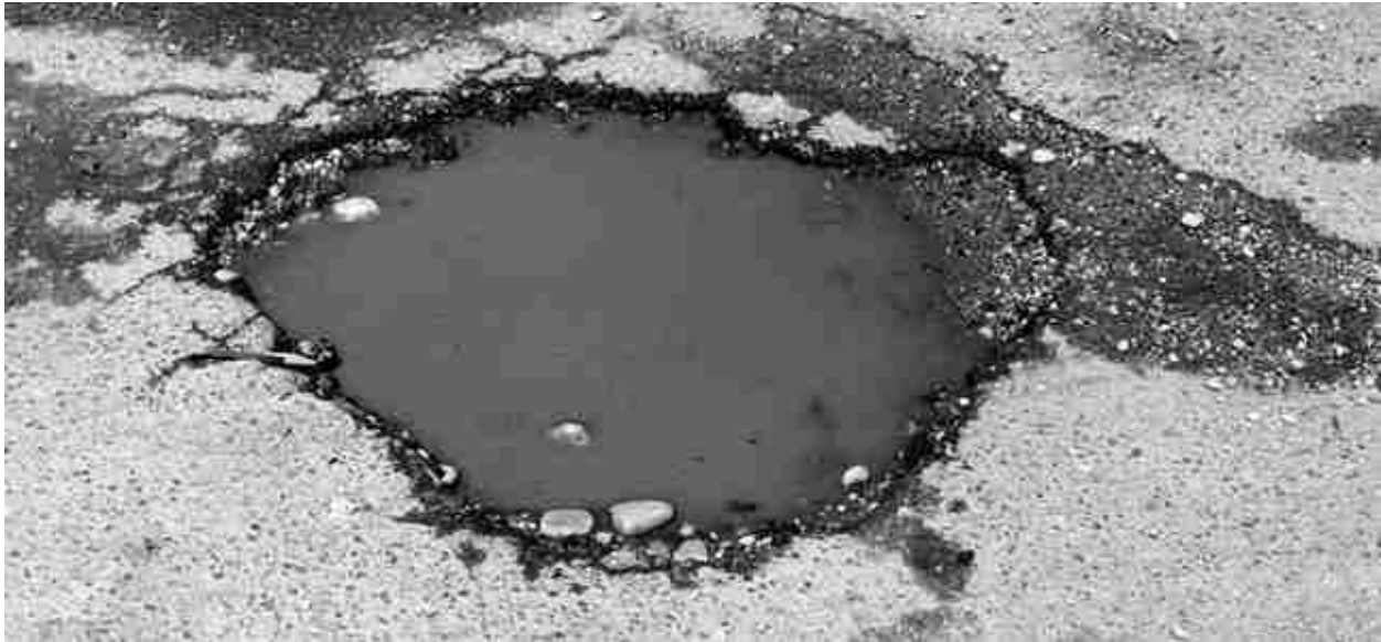
Figure 2.2: Moisture damage (stripping) [16].
