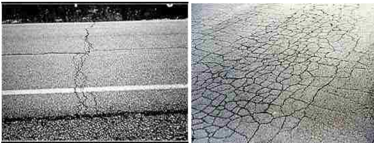
Figure 2.4: Thermal cracking of asphalt pavement [22,23].
