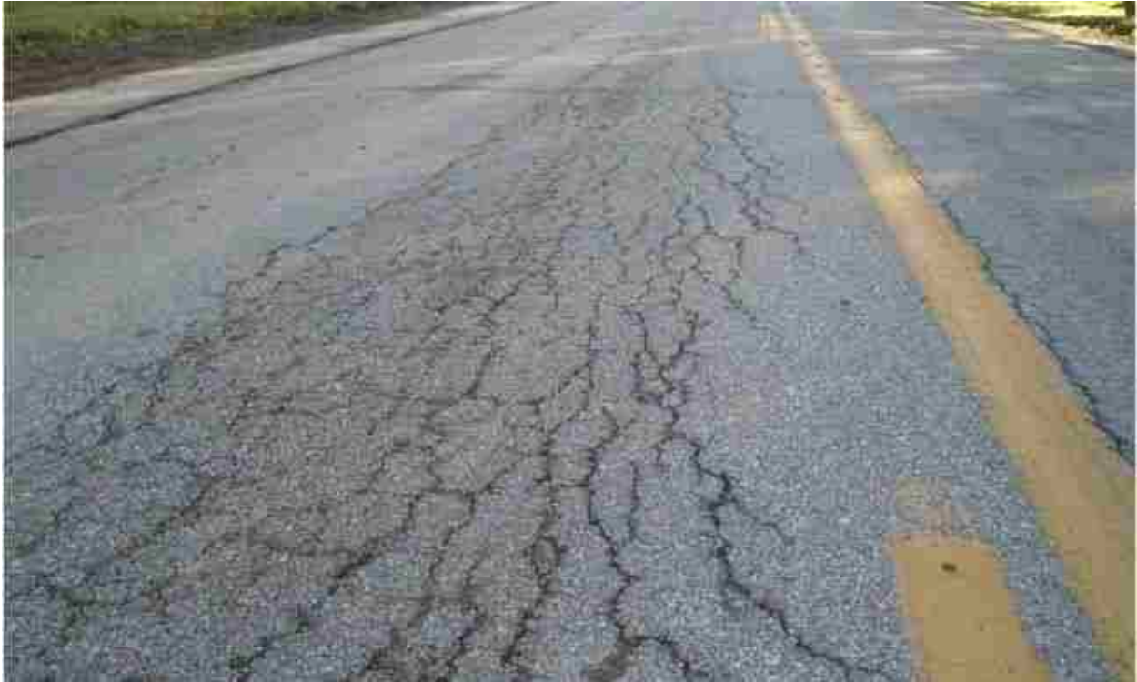
Figure 2.1: Fatigue (alligator) cracking [15].
