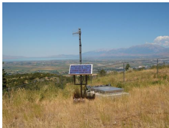
Figure 2.4 – Automated chemical release and monitoring remote terminal unit (RTU) station. Powered by photovoltaic and long range communication via directional radio antenna. In a field on a hill. Image by Dan Steele, 2012.
