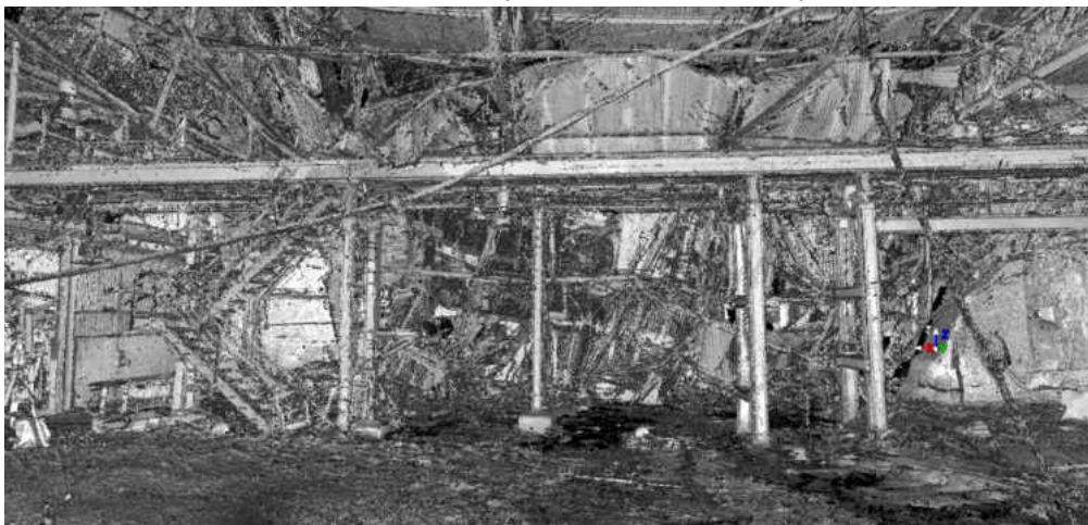
FIGURE 2.13: Brymbo ironworks foundry, collapsed roof
