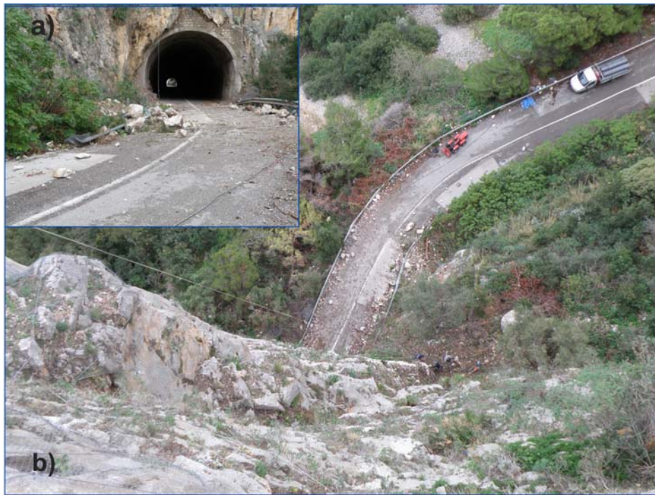
Figure 4. Examples of rock-fall in a main road in northern sector of the study area: (b) rock-fall release area and (c) rock-fall deposits.
