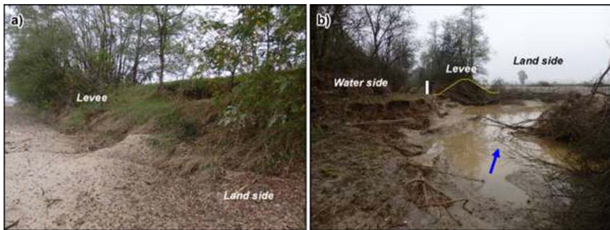
Figure 7. Damage to the levee system at Garzaia. (a) Structural damage to the levee embankment. (b) Levee breach and scour hole; the dotted line represents the levee cross section and the blue arrow indicate the main flood-water direction. The vertical white line represents a real height of 2.2 m.
