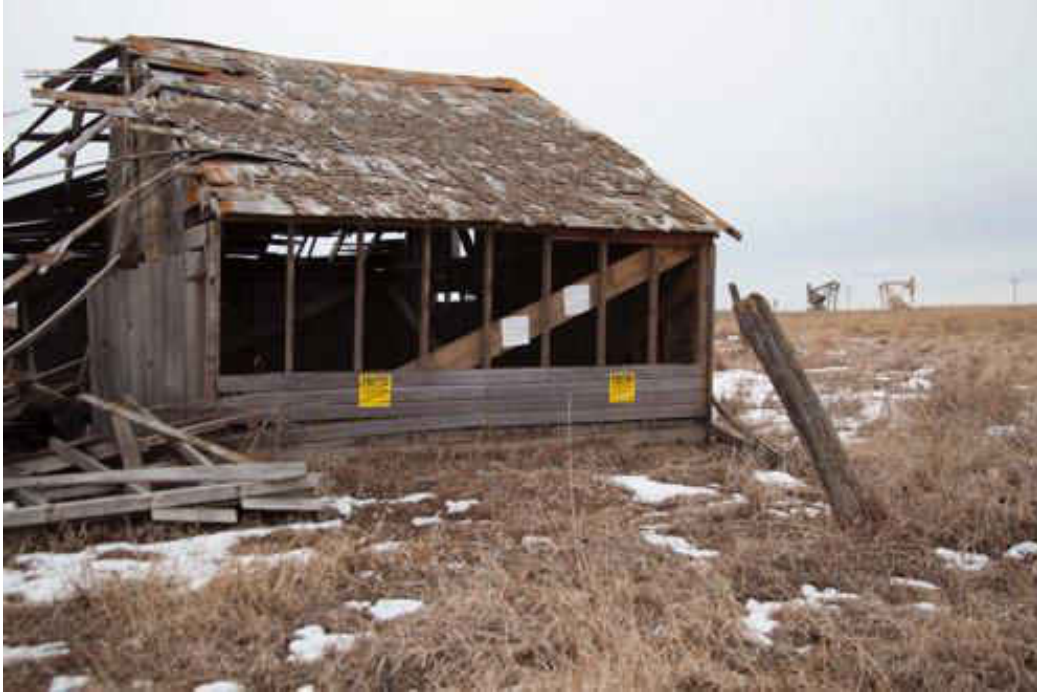
Figure 54. Historic barn on the homestead of Phoebe's father. According to Phoebe, the barn has collapsed from the winter snow load and dismantling by craft enthusiasts.
