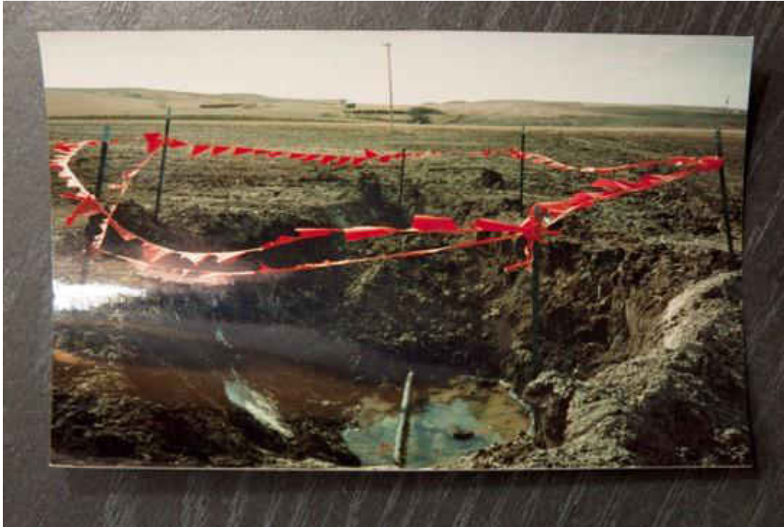
Figure 12. Pipeline break. Image made by Cody on his land on March 18, 1992.
