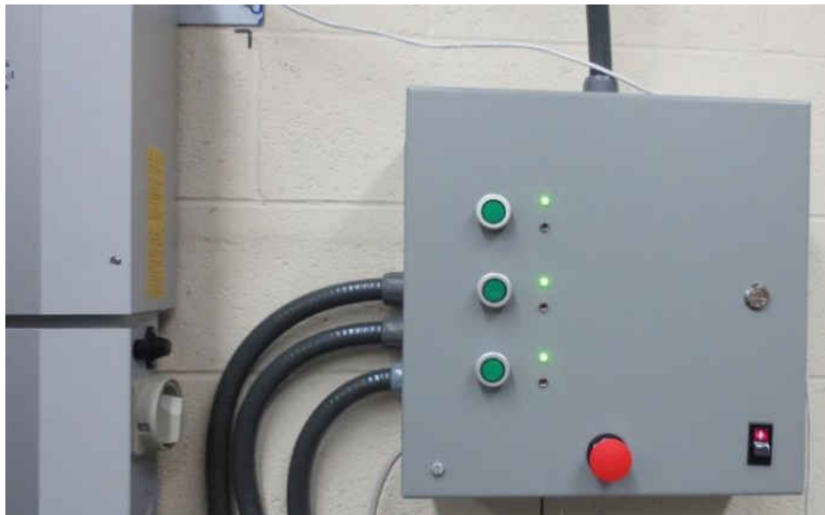
Figure 3.14: PV load switching enclosure.
