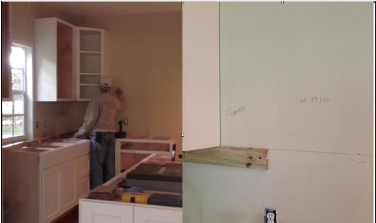
Figure 13: Ned transfers measurements from the CAD drawing to the wall prior to installing a cabinet piece.
