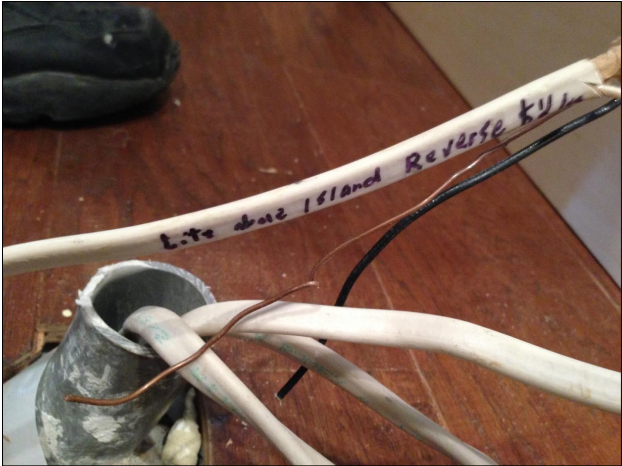
Figure 15: The electrician annotated the wiring so that other subcontractors would see each wire's function.
