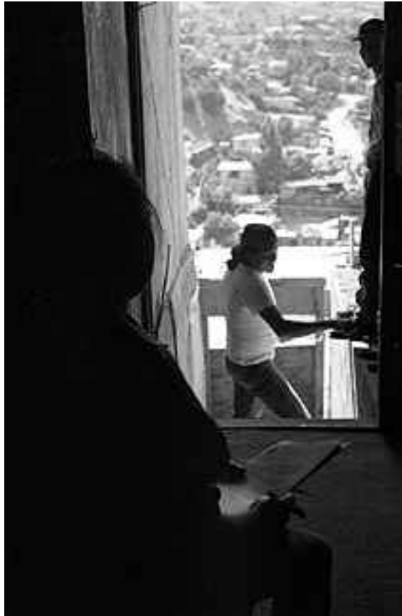
Figure 15: A room in Delfina's house, under construction. Photo by Luz Aida Ruiz Martinez, Grupo Factor X
