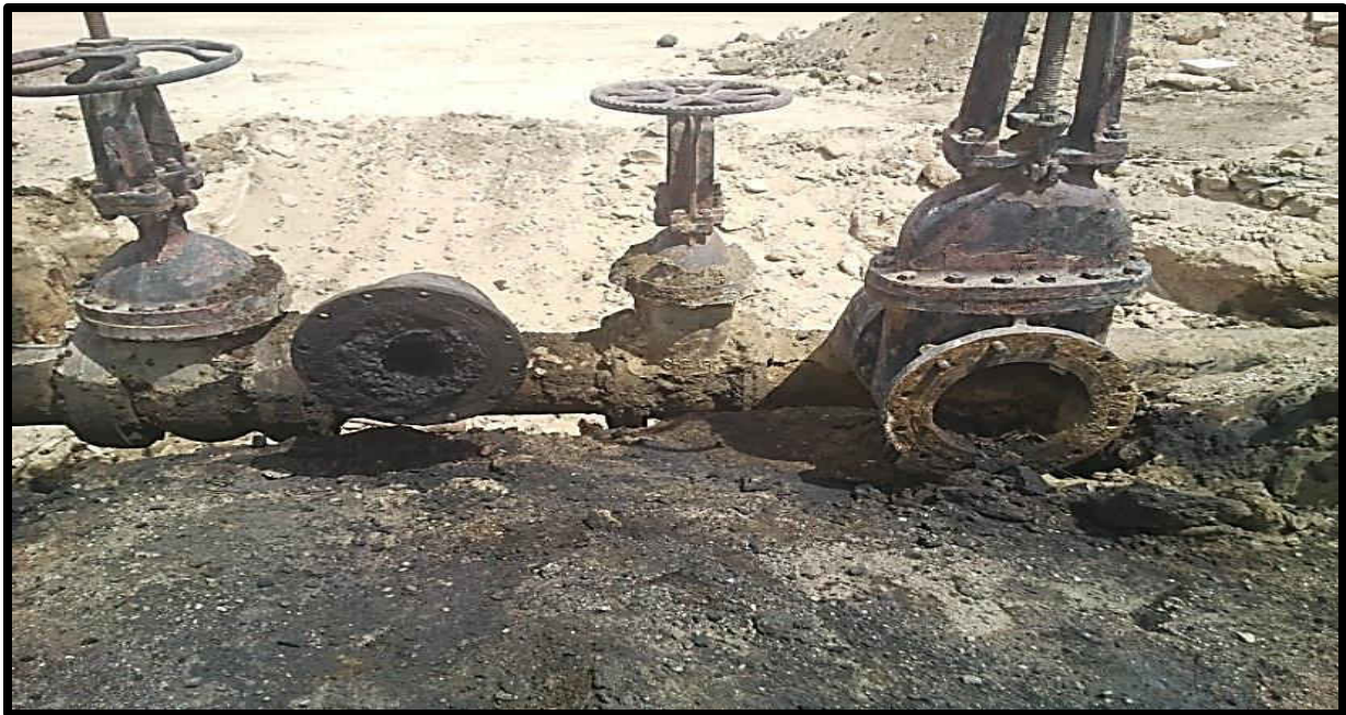
Figure 4. 16 : Valves Contain Scales and Accumulated Deposits
