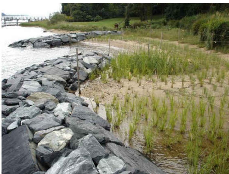
Figure 26 A "living shoreline" that is actually a hard stabilization (concrete rip-rap) with Spartina alterniflora planted landward in Edgewood, Maryland.
