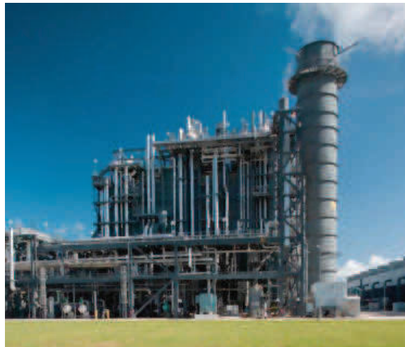
Figure 2.1: OUTSIDE VIEW OF HEAT RECOVERY STEAM GENERATOR
