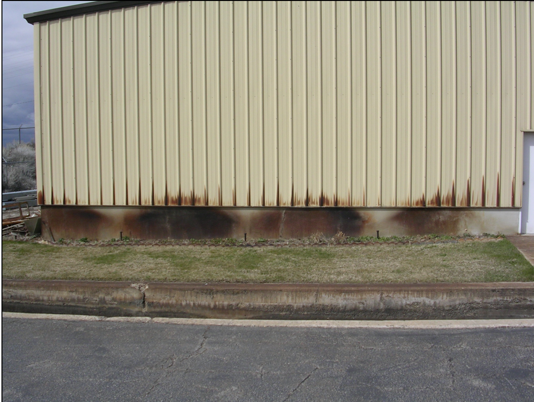
Figure 3. Ferric staining on city-owned structures.
