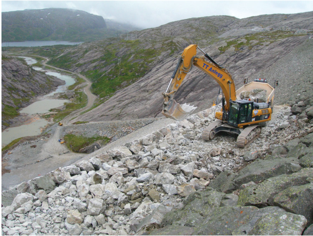
Figure 1 Reconstruction of a placed single-layer riprap on the downstream slope of the 129 m high rockfill dam Svartevatn in south-western Norway. The riprap stones are placed one by one in an interlocking pattern and form with the adjacent filter layer an erosion protection against accidental leakage and overtopping. (Photo: NTNU)
