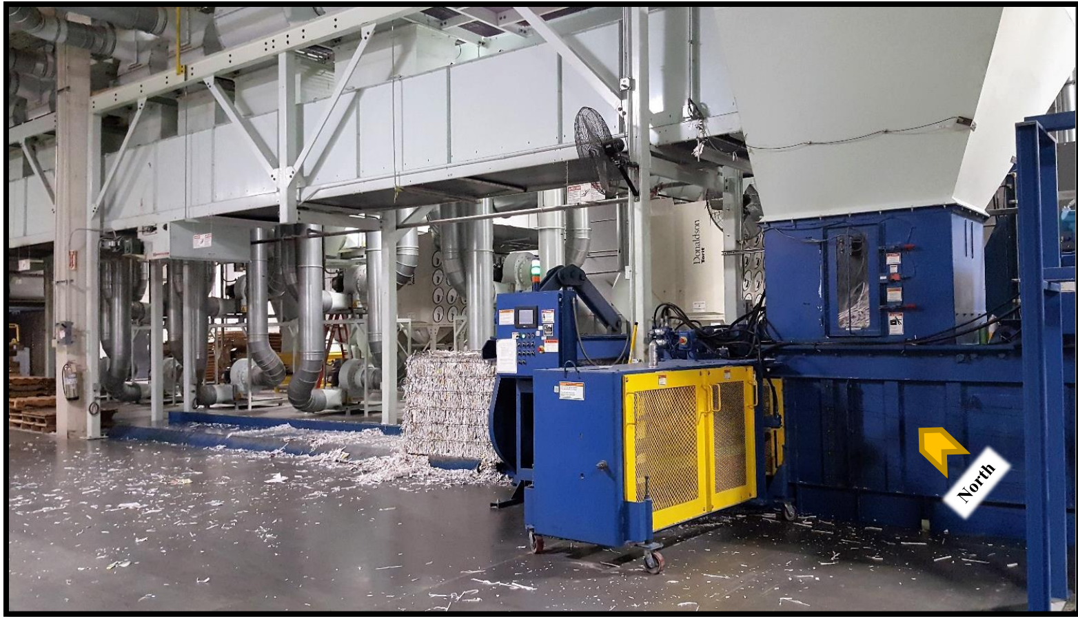
Figure 4. The Baler Room work area.
