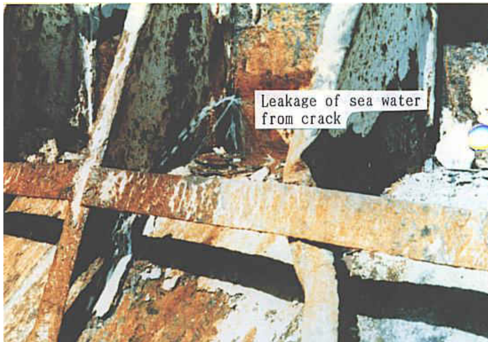
Figure 4: Leakage from side shell plating due to heavy corrosion
