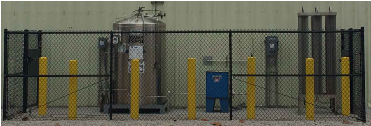
Figure 2.12: CO 2 microbulk tank with electric and ambient vaporizers
