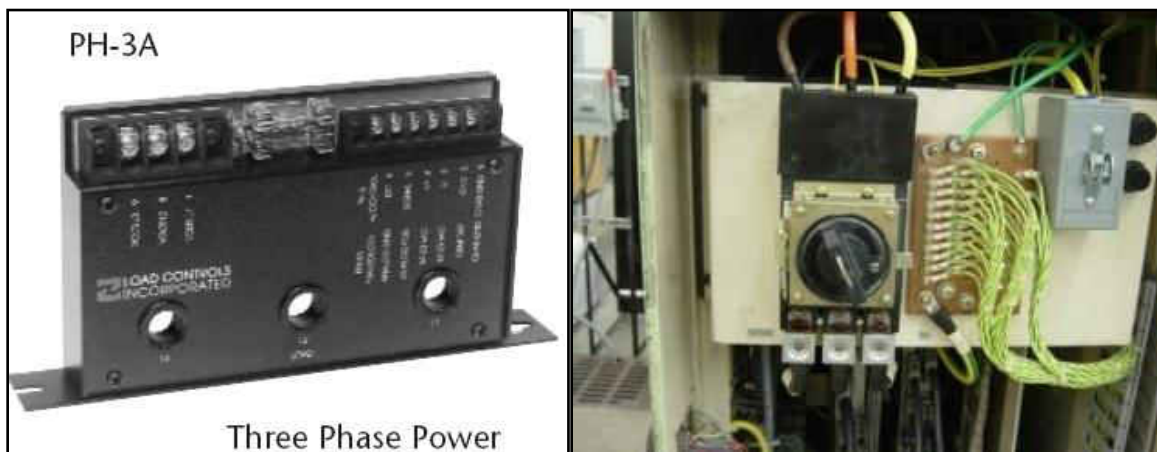
Figure 16: Power Meter in Electrical Cabinet
