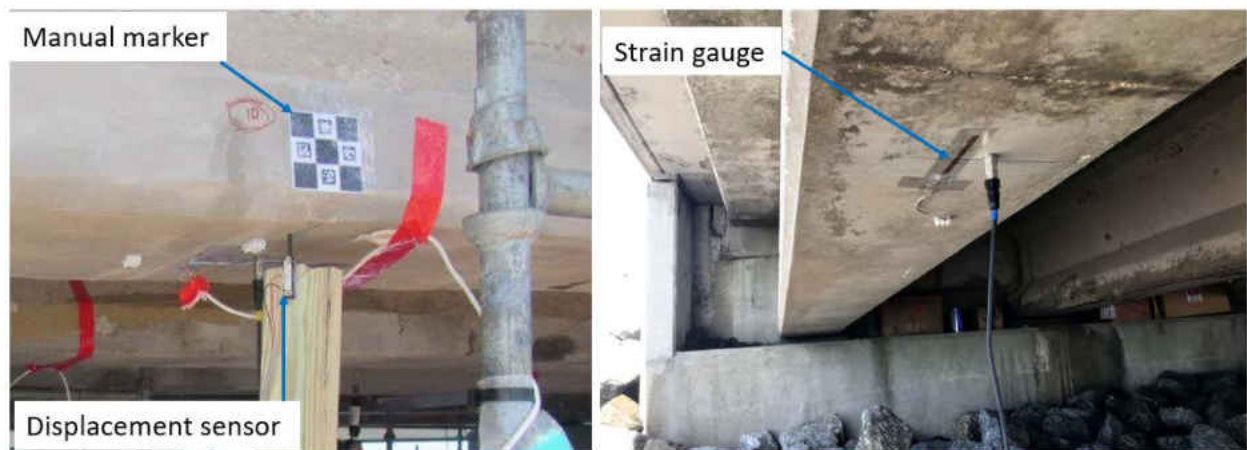
Figure 105 Sensors installed on the bridge
